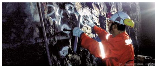
DSI Undergroup, DYWIDAG-Systems International (DSI)
